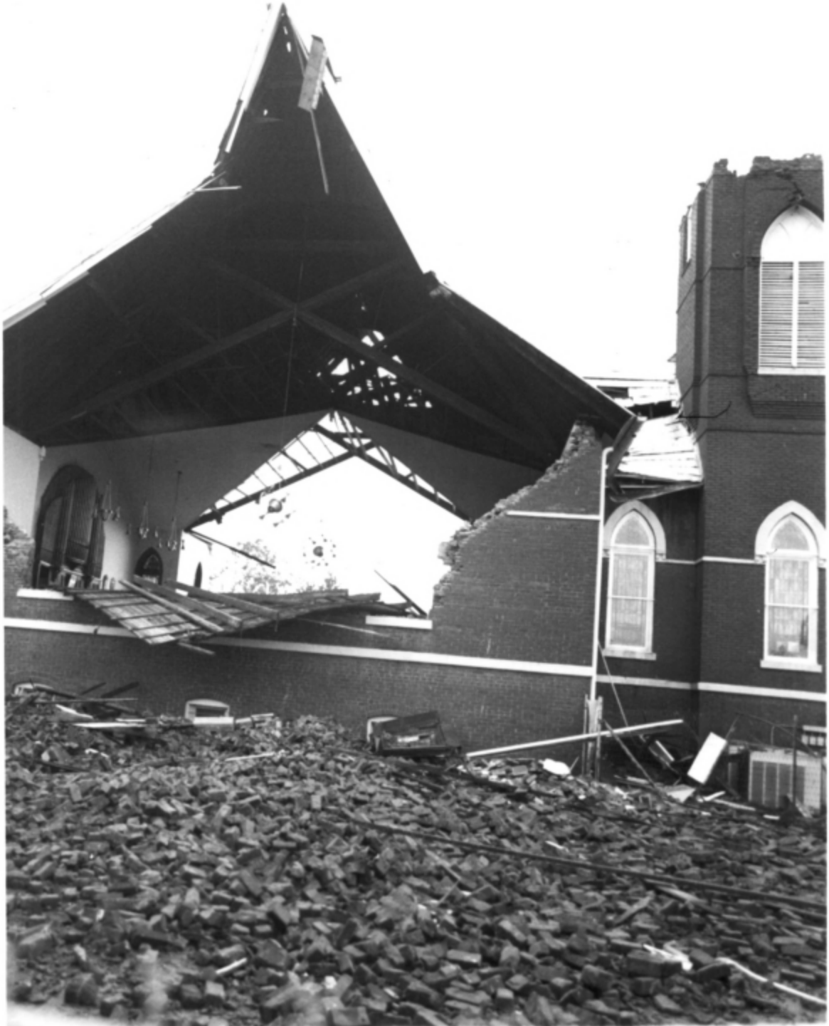
South wall, showing tornado damage. This photograph part of the National Register nomination for First Baptist Church. Selma Times Journal 1978. Mertins 1979).
