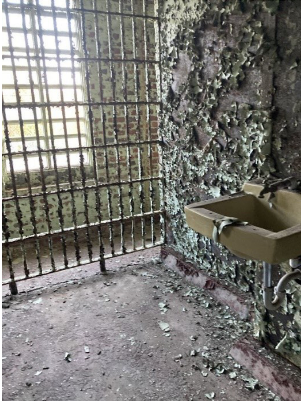
Interior of Old Perry County Jail. First floor individual jail cell. NPS study team 2022.
