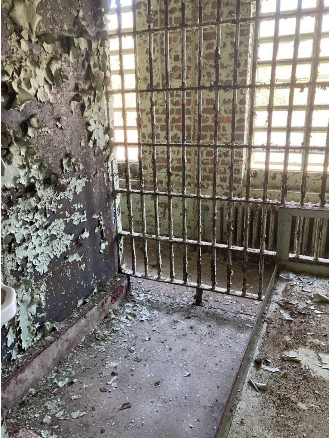
Interior of Old Perry County Jail. Jail cell on the first floor where Reverend James Orange was held. NPS study team 2022.
