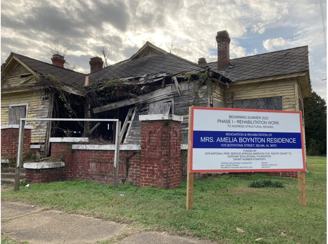
View of the front of the Boynton Home and rehabilitation project information. NPS study team 2022.
