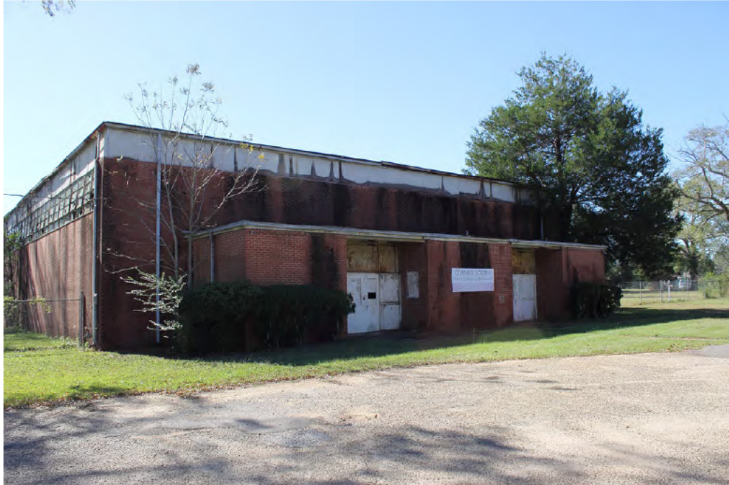
Gymnasium. The photograph is part of the National Register nomination for the Lincoln Normal School. Causey 2020 in Pope Burns and Van West 2022.
